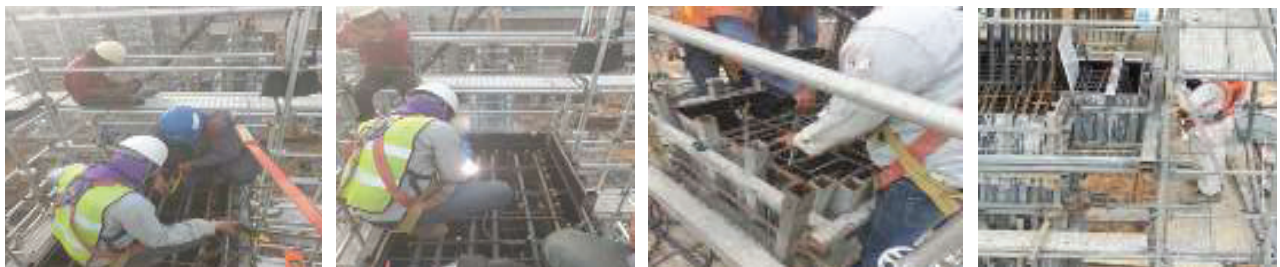
Figure 1 The setting anchor bolts use the electric welding cabinet. (before improving the work process.)
