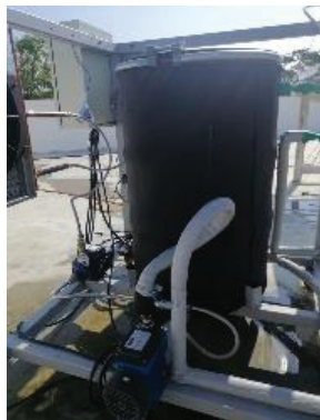
(c) Storage tank
