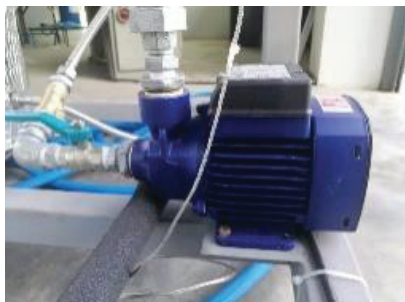
(e) Water pump
