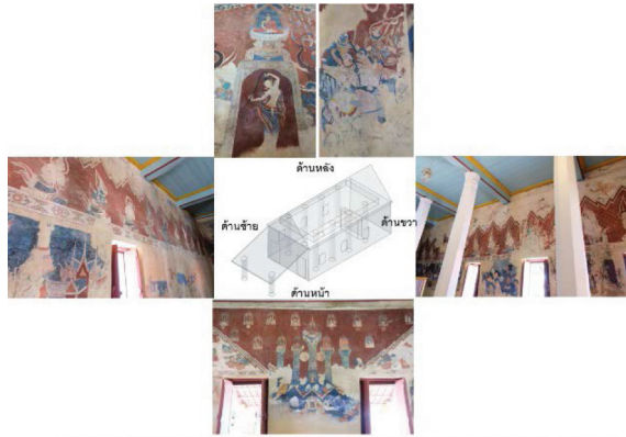
Figure 7 The Damaged mural painting inside the Ordination Hall, Wat Chang Yai
