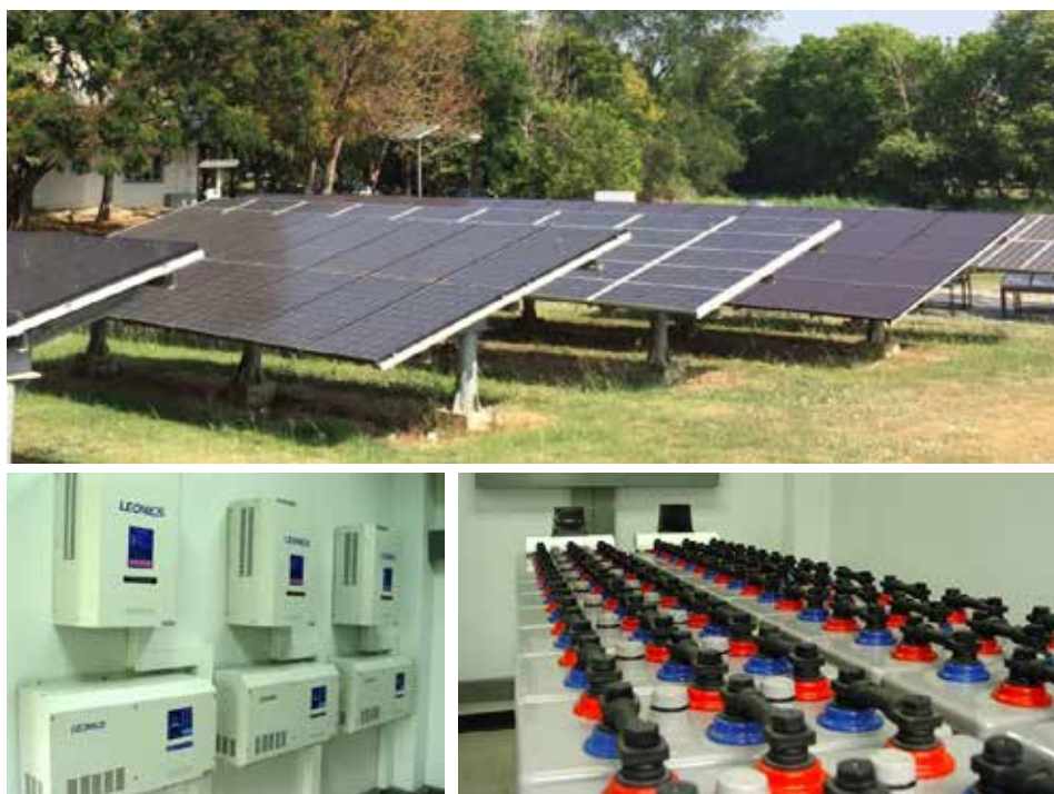
Figure 3 10 KW PV system at the energy park, School of Renewable Energy Technology (SERT), Naresuan University, Phitsanulok, Thailand.
