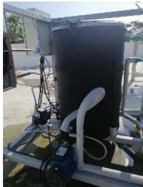
(c) Storage tank
