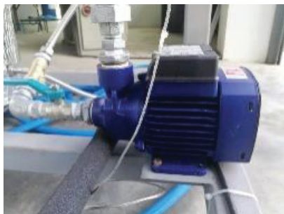
(e) Water pump
