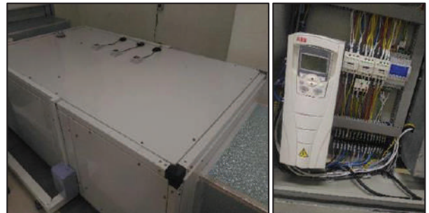
Figure 7 AHU and VSD set
