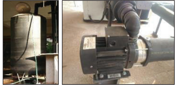
Figure 6 Chilled Water Storage Tank and Chilled Water Pump
